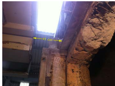
Burner trolley rails overhead close to the doors.
