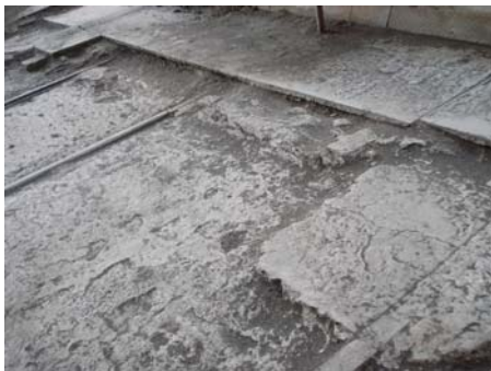
Uneven floor in front of the kiln hood.
