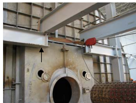
Burner trolley rails overhead.
