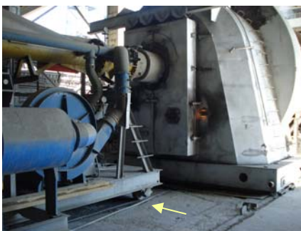
Burner rails in the floor in front of the kiln hood.
