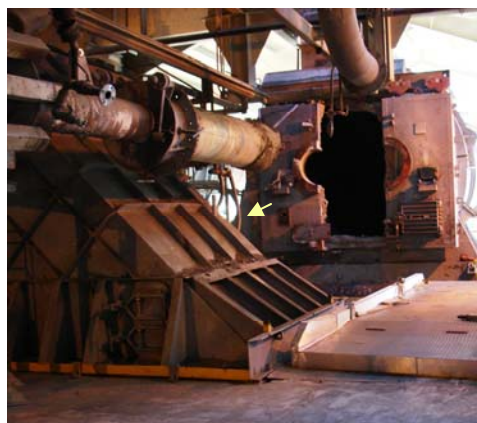
Tertiary in front of the door and burn tube not retractable.
