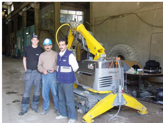
From left to right: Brokk supervisor Mattias Lundmark together with Mr. Habibi, head of Operation Dept. of Neka Plant, and Mr. Sadrollahi, Operator of the Brokk machine.
