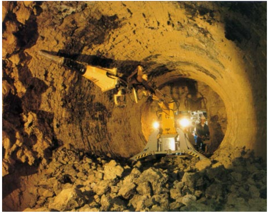
Some 25 metres (985 in) of coating and bricks were demolished by a Brokk 250 and one skilled operator, during only three hours of effective working time.
