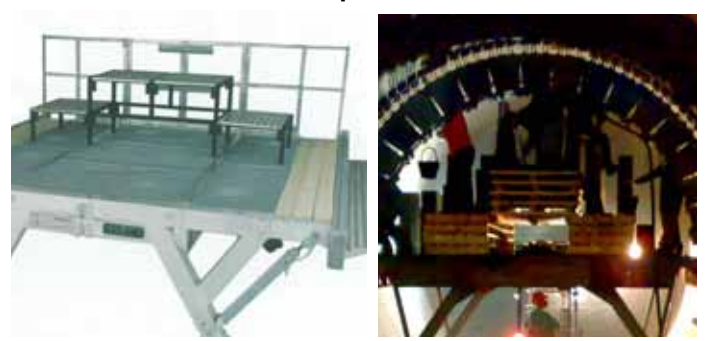
A stair step "drag along" jump scaffold serves a work platform with no safety rails on the scaffold itself
