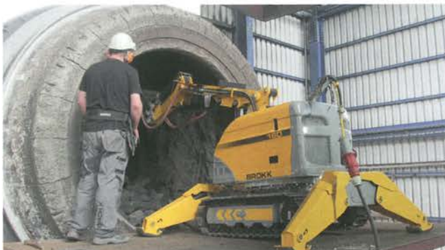
Remote-controlled demolition machines are the safest and quickest way to remove refractory brickwork.
