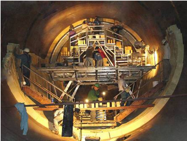
Large Flat Deck machine at the Tilden/Cliffs plant
