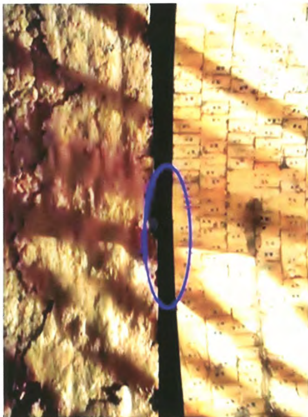
Figure 2. Distortion in brick alignment at the cut row.
