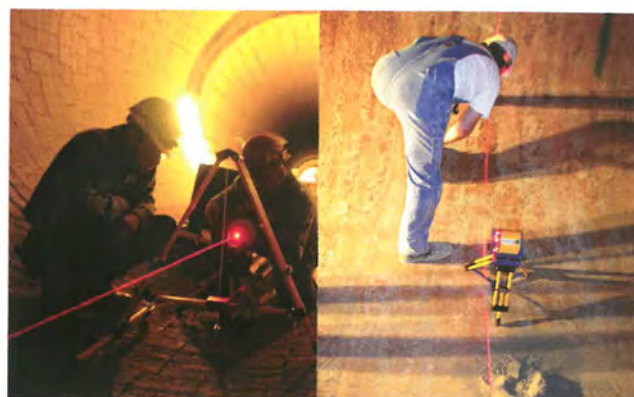
Figure 3. Radial laser ensures the bricks are properly aligned; guidelines can be marked and reproduced at several points along the kiln.
