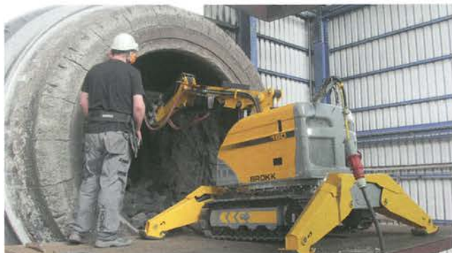
Remote-controlled demolition machines are the safest and quickest way to remove refractory brickwork.
