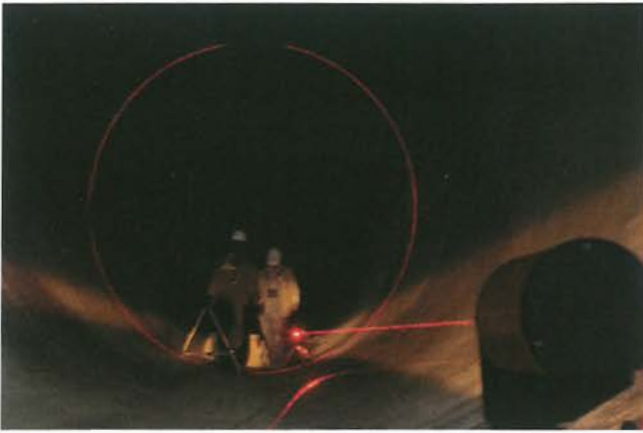
A laser alignment device gives masons a point of verification throughout the entire length of installation, ensuring proper radial alignment of the refractory.
