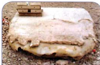
Typical damage to a conventional design of TAD with castable refractory.
